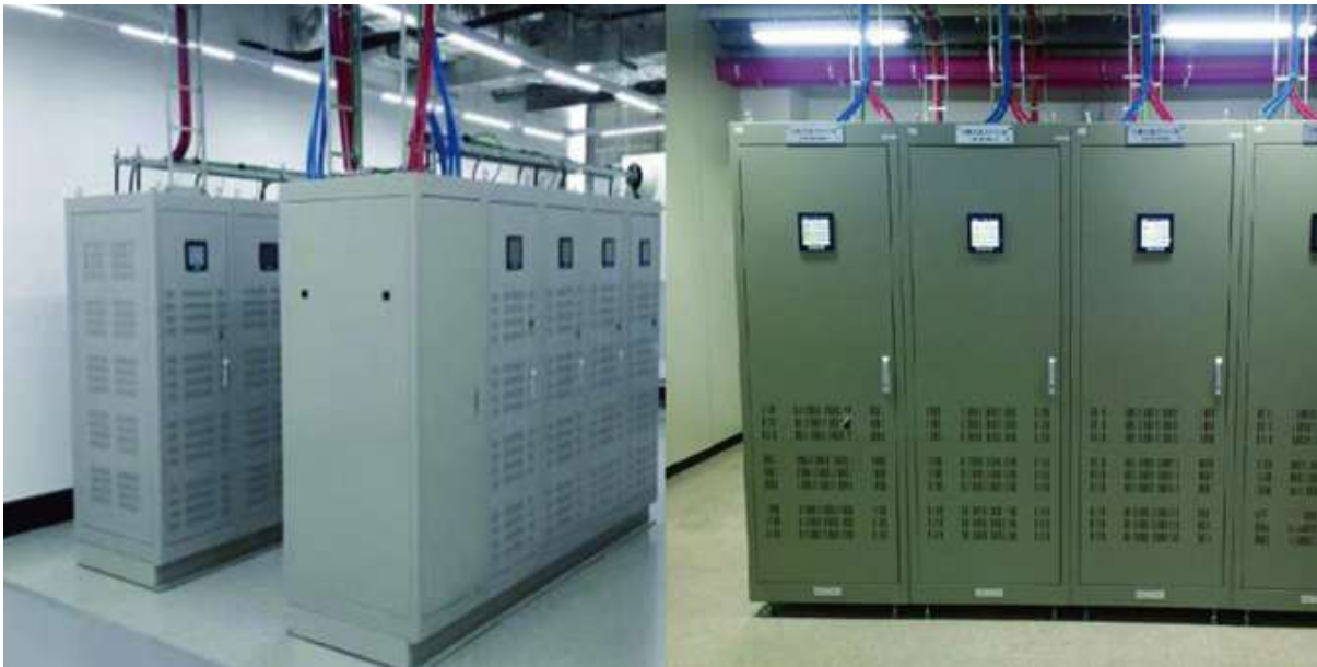
South Korea IDC Data Center Project
