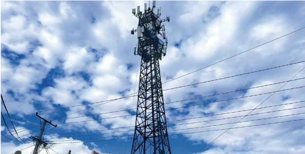
China Mobile Heilongjiang Smart Sodium Battery Project
