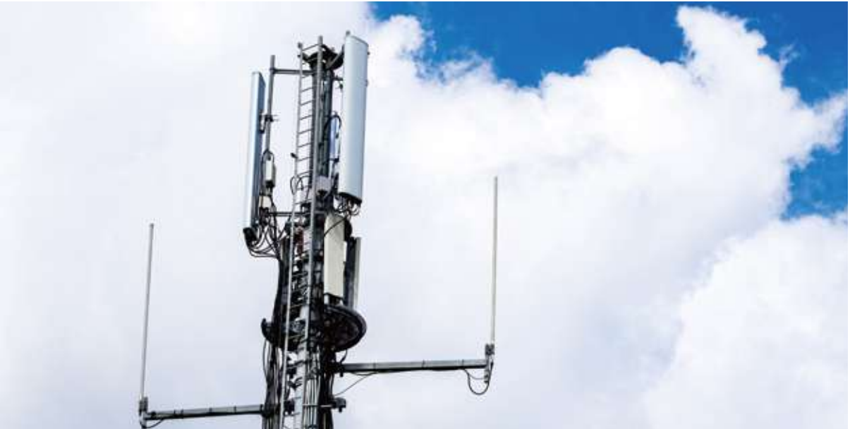
China Tower Heilongjiang Smart Sodium Battery Project
