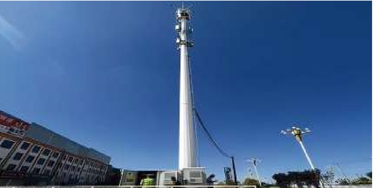
China Tower Gansu Smart Sodium Battery Project
